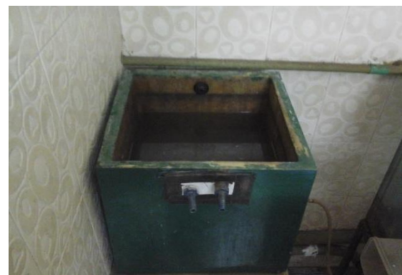
Fig. 5. Sodium Chloride Solution tank (5% NaCl)
