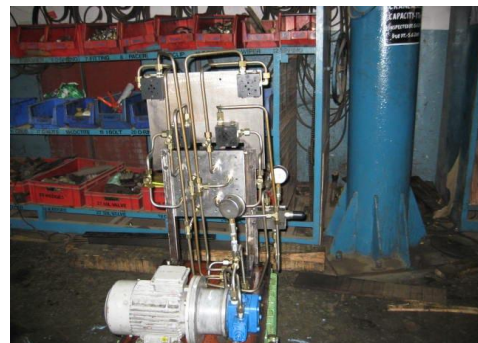
Fig. 2 – Hydraulic Power unit (After)
