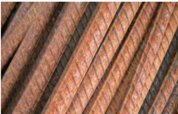
Fig 4 Overall view of #3 bars left exposed outdoors
