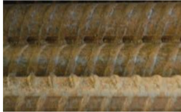
Fig 7 The tight rust has not altered the deformations Left exposed to normal atmospheric Conditions on the #9 bar surface.
