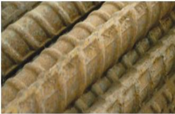
Fig 6 Tightly adhered rust on a bundle of #9 bars for 22month
