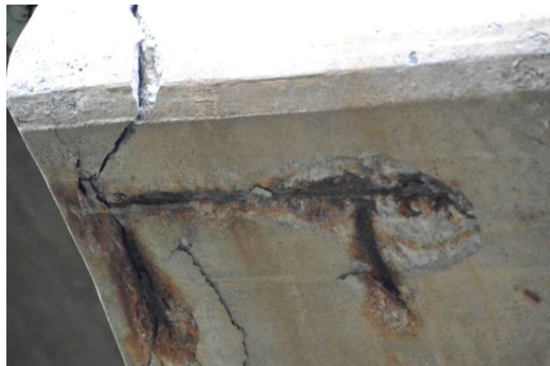
Figure 10 –Corroded steel Reinforcement possibly due to insufficient concrete cover
