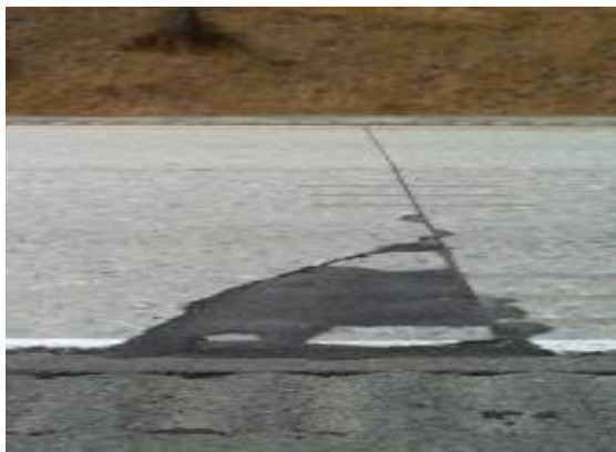
Figure 8 Failure of Joint load Transfer system
