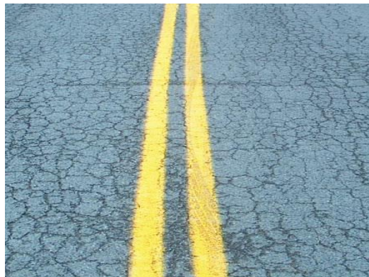
Figure -1 Flexural fatigue cracks
