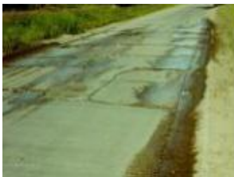
Figure 2 Pumping in rigid pavement
