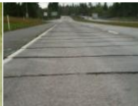
Figure 3 Faulting in rigid pavement
