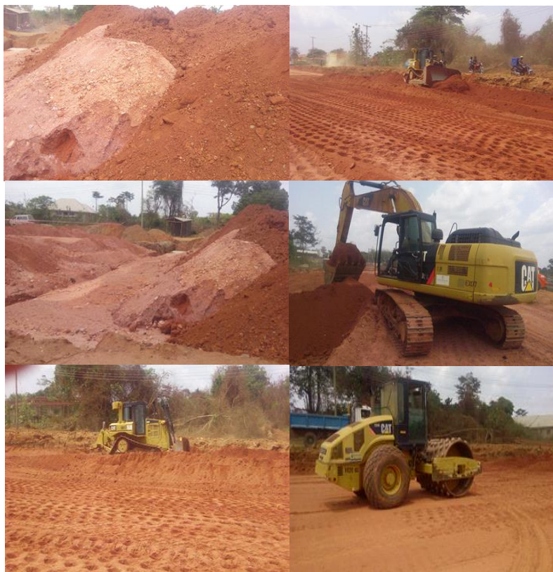
Fig. 2 Some of Site photographs taken along the roadway showing different construction processes and machine/equipment.
