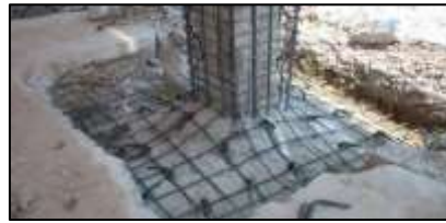
Figure 8: Plain Concrete in the Extended Area and the Reinforcement Bars Arranged Surrounding the Footing.
