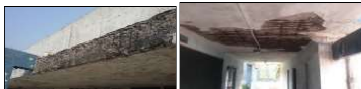
Figure 6: Bldg. shows Exposed Reinforcement. Figure 7: Spalling-Off Concrete Observed on Ceiling
