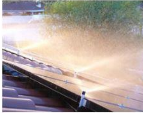
Figure 15 Heliotex sprinkler system
