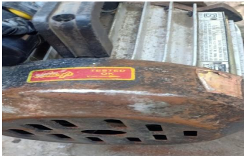
photo-rusted cover of industrial water Before treatment
