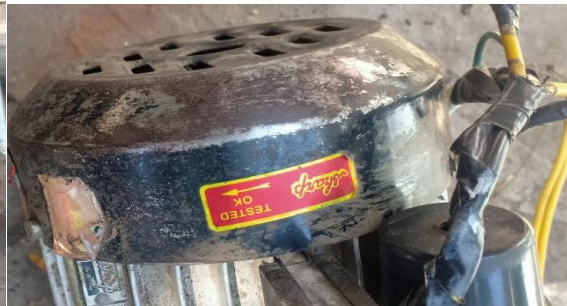
photo clean cover of industrial water pump after treatment with RSP metals
