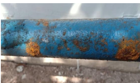
Photo showing Rust deposition on company
