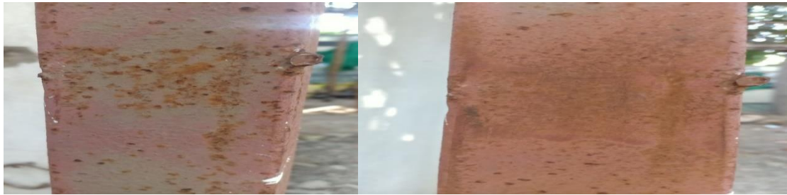
photo heavy rust on Primer coated pipe
