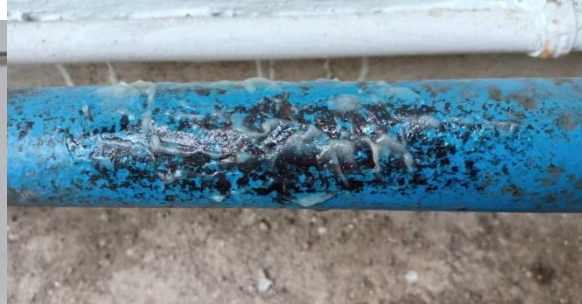
photo :- water supply Pipeline in chemical plant applied with rust prevention paste
