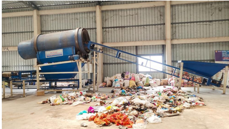
Fig. 4: Dry waste segregation machine in Kagal MSW plant
