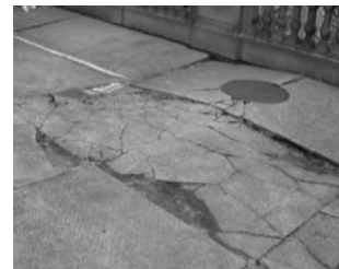
Heaving concrete cracks
