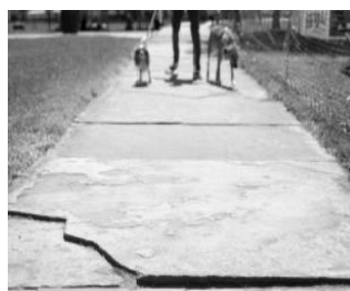
Expansion concrete cracks
