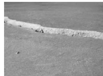
Settling concrete cracks
