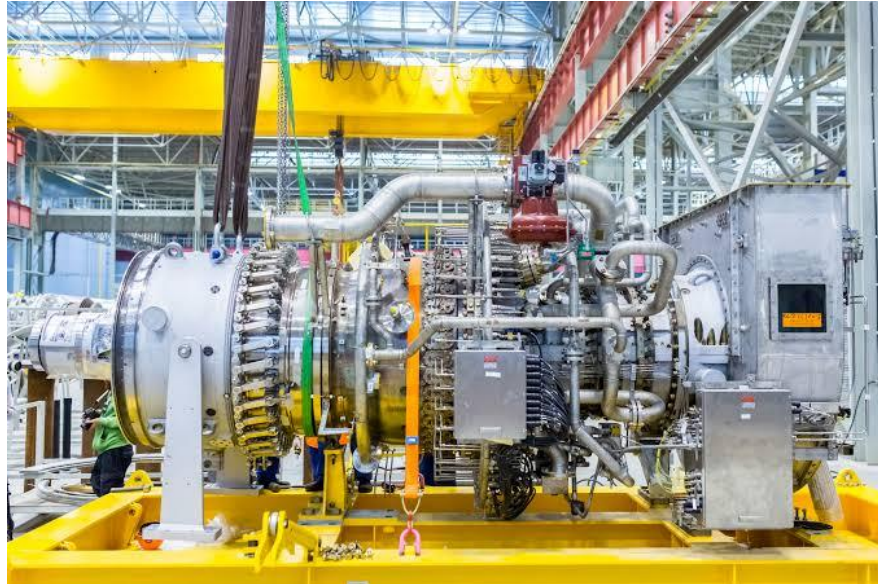
Figure 1B: Gas turbine in Afam power plant.
