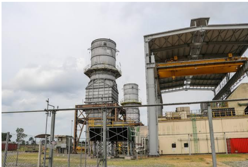
Figure 1A: AfamVI Gas power plant/first independent power Ltd
