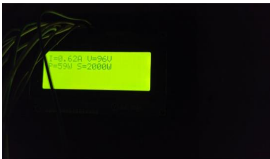
Fig8.1 Energy Monitoring System Result Displayed
