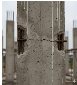
Fig. 3. Finishing defects in RCC.
