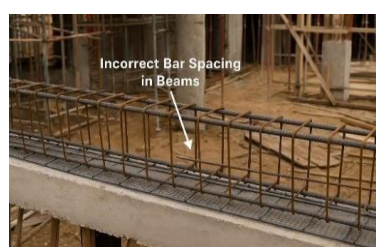
Fig.1 Improper Bar Spacing
