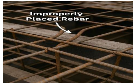
Fig.5 Poor Reinforcement Placement
