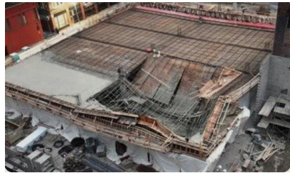
Fig.3 Formwork failure during slab construction (13)
