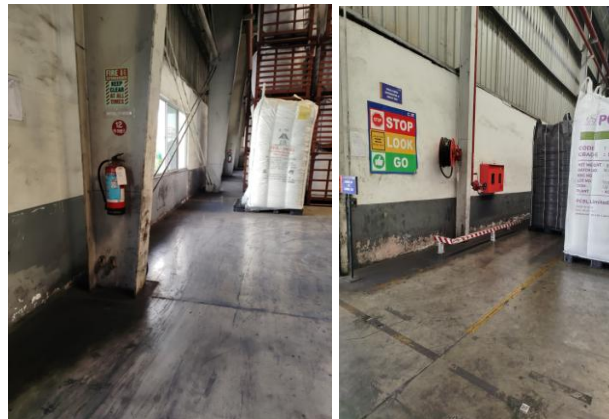
Fig. 8. Fire Extinguisher & Fire Hydrant for fire fighting
