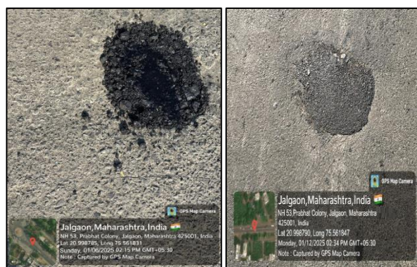
Figure 3: Pothole repaired using modified bitumen mix (immediately after repair and after 6 months)
