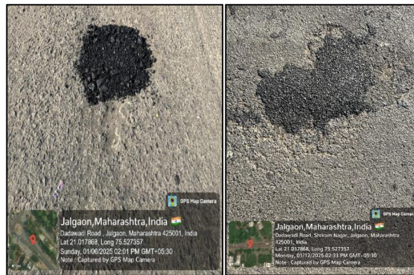
Figure 2: Pothole repaired using conventional bitumen mix (immediately after repair and after 6 months)
