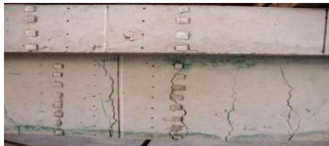
Fig 4.2: Control beam after cracking
